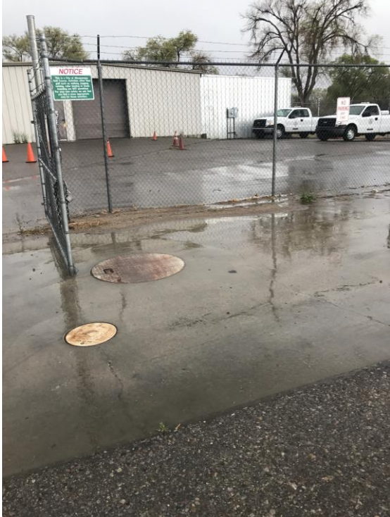
Photo 1: Water pooling on site coming from golf course storage shop.
