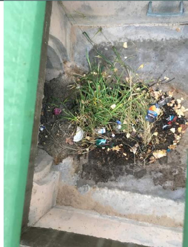
Debris observed in Outfall LGC1
