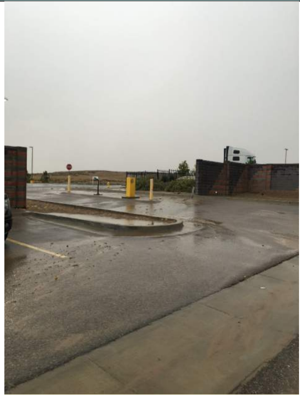
Some evidence of erosion near employee parking lot.
