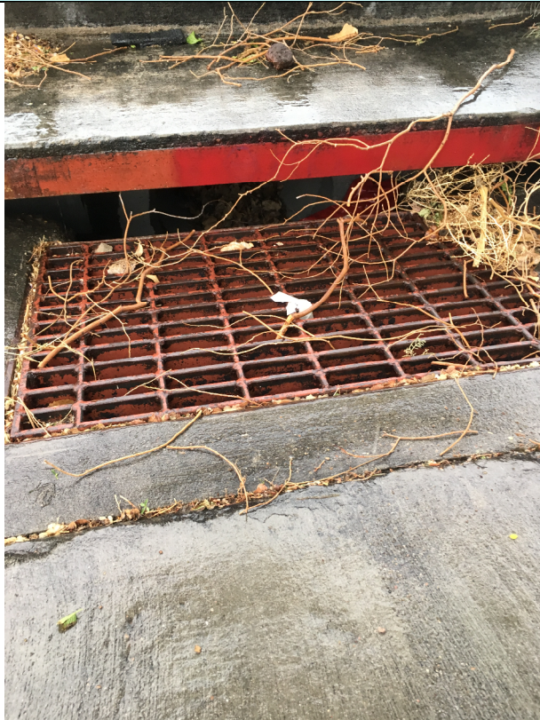
Photo 1: Outfall PDS1. Leaves and debris observed in outfall.
