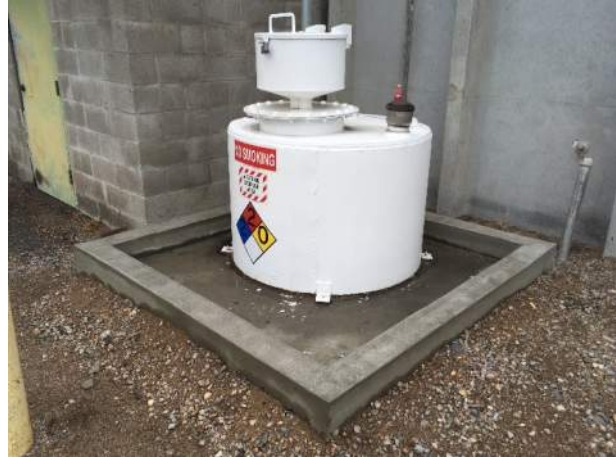
New containment provided for used oil tank.
