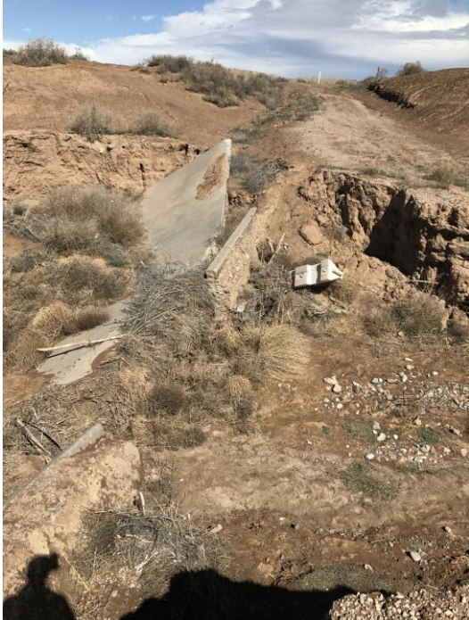
Destroyed Outfall MP2
