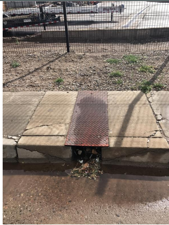
Photo 2: Leaves and some litter observed in AM1 outfall.
