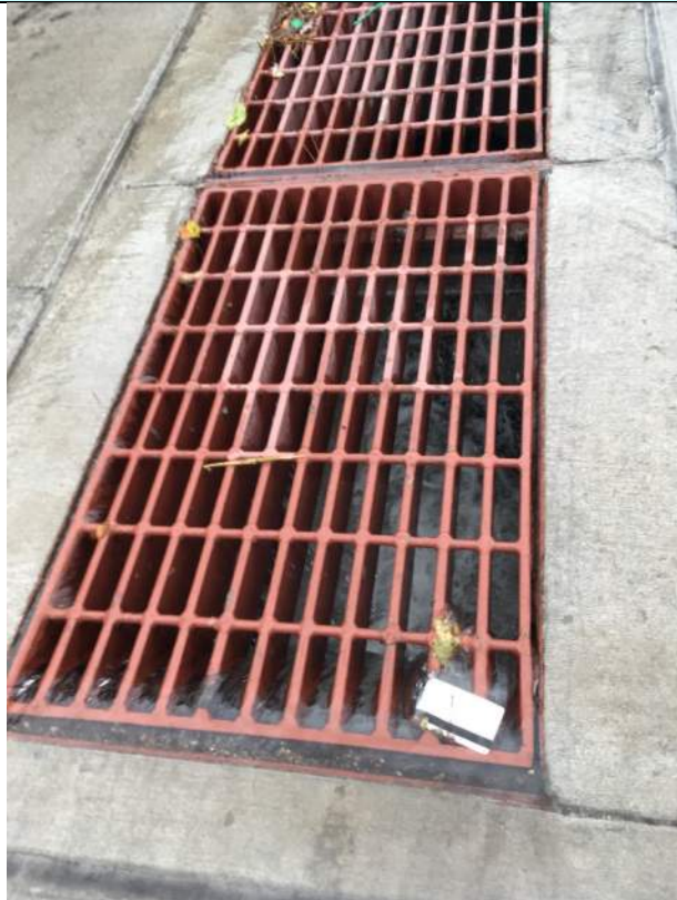
Flow observed entering water quality structure inlet structure.
