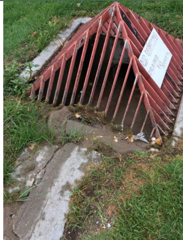
Evidence of grass clippings and sediment entering outfall.
