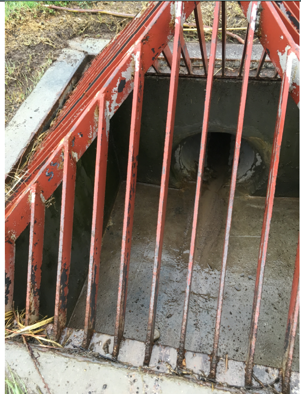
Photo 2: Outfall PDS1. Debris has been removed from outlet since last monitoring event. No apparent storm water quality issues.
