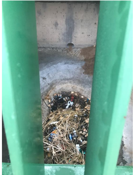
Debris observed in Outfall LGC1
