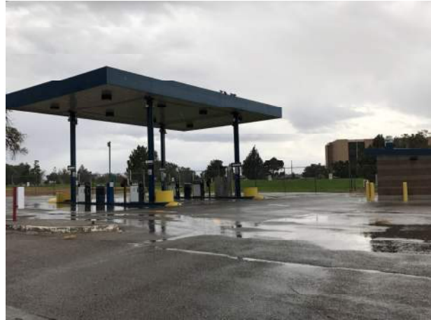
Outfall L1: No apparent impacts to stormwater quality apparent in pooled runoff.
