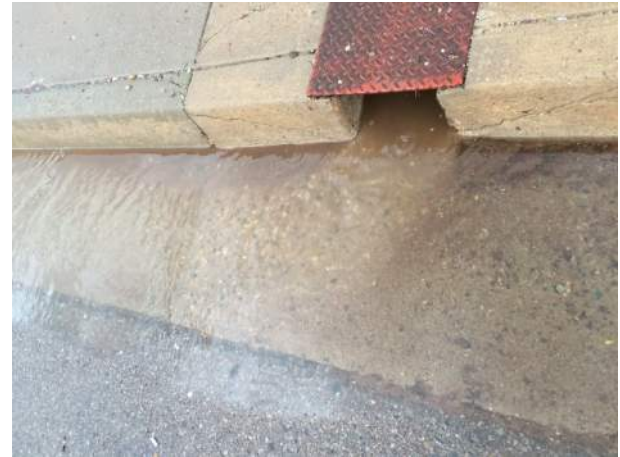
Runoff observed in curb.
